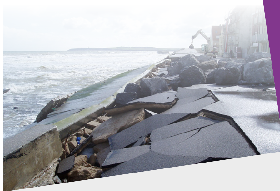
◀ Complete destruction of a section of road after a storm.
