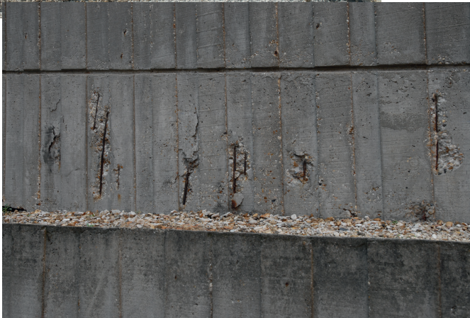
▲ Example pathologies (spalling) of reinforced concrete due to reinforcement corrosion induced by carbonation.
